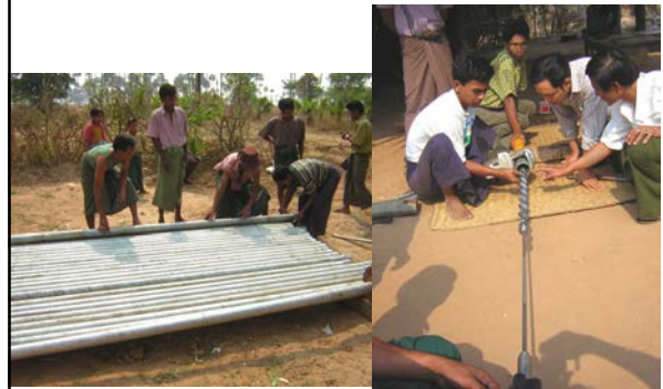
Checking and preparing the riser pipes and mono element for pump installation at Htantawgyi village
