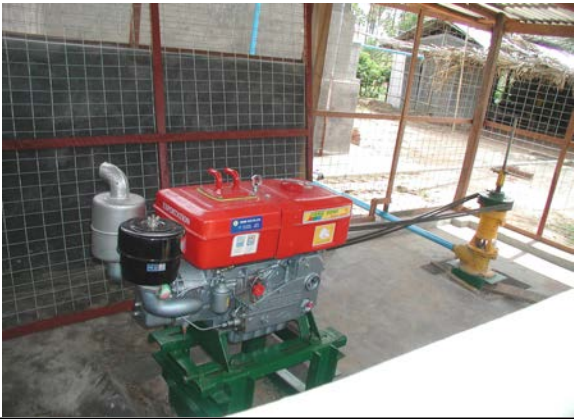
Engine installed at Htantawgyi tubewell
