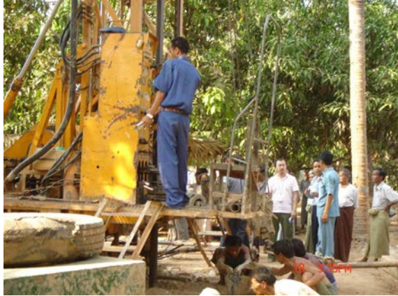
EOJ mission and DDA officers studied well drilling process at Twinma village
